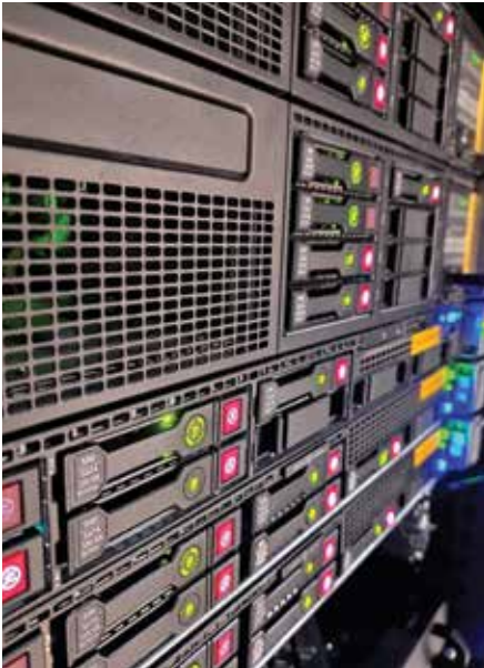
Server room, Odisee University College, Ghent campus
