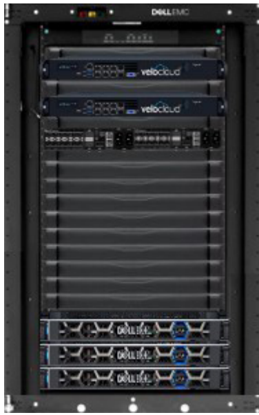
FIGURE 2. VMware Cloud on Dell EMC infrastructure rack
